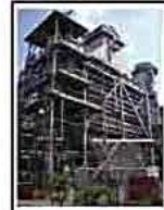
Gas Turbine Inlet Pre-cooler
